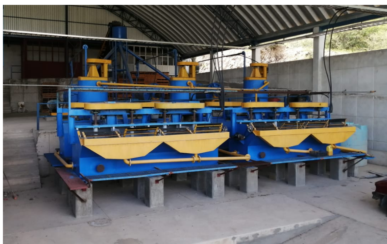
Figure 1. Flotation Cell Banks at Tecmatlán
