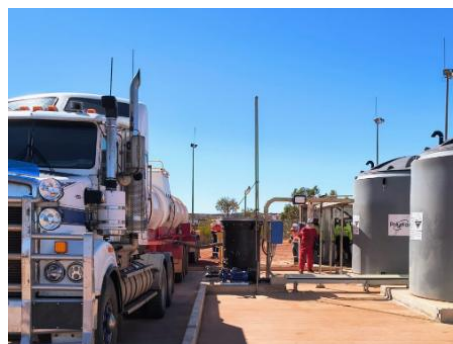
Acid terminal receiving first acid delivery
