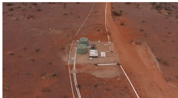
Figure 7: Siphon raw water borefield
