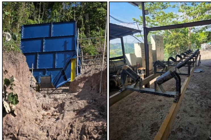
Photos 8 and 9. Coarse Ore bin complete assembly and conveyor belt.
