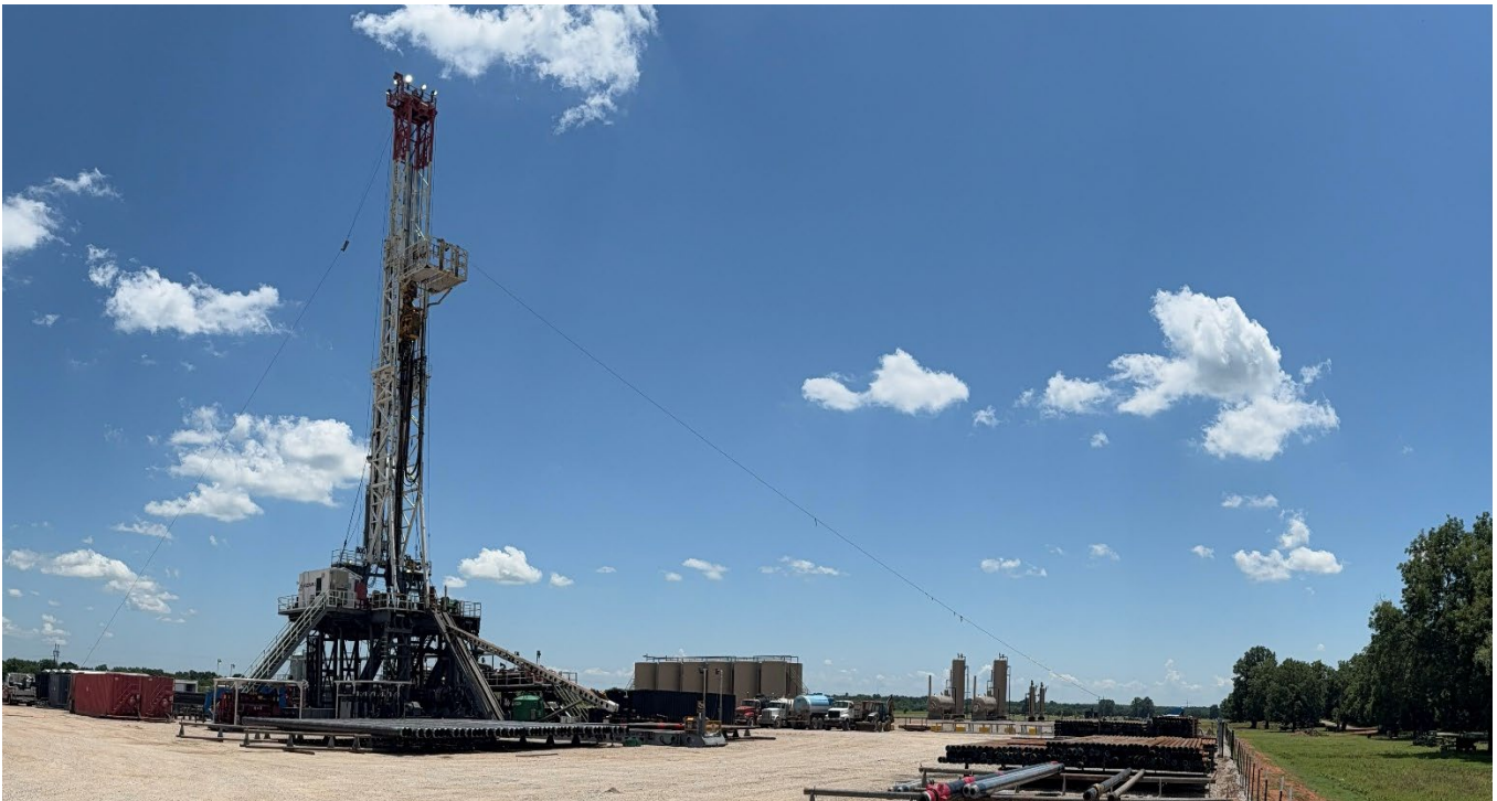
Kenai Drilling Rig 18 on the Suttles pad in the SWISH AOI, Oklahoma with production facilities, including tank battery and separators in the background.
