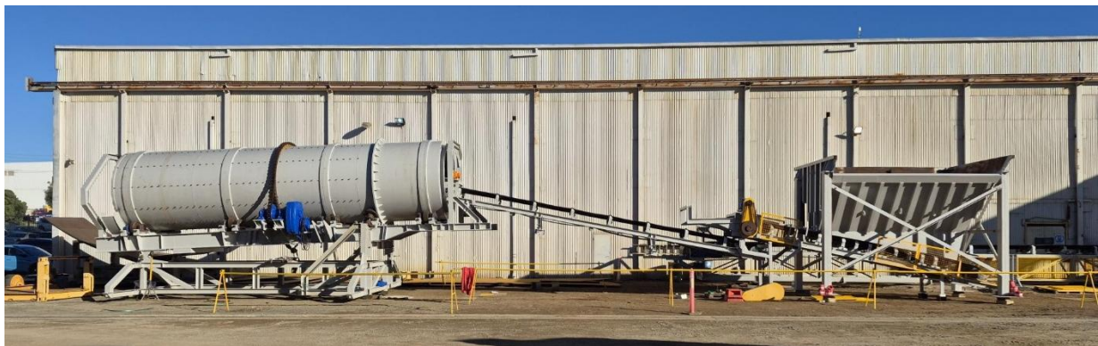
Figure 1: OZM feed bin, feed conveyor and agglomerator drum at Polaris Engineering Services Henderson Facility
