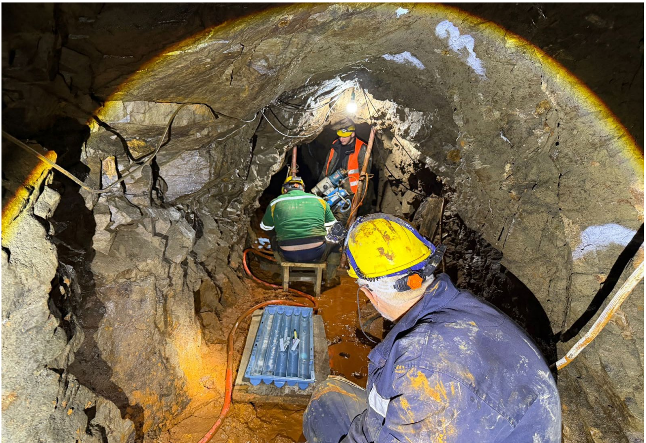
Figure 1 Drilling setup in operation in Adit 51 on Vein 10. Samples in this area have returned high grade Sb results (refer to ASX announcement 13.02.2025)
