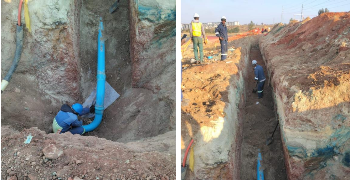
IMAGE 3: INSTALLTION OF POTABLE WATER INFRASTRUCTURE WHICH INCLUDES CONNECTION TO MAINS WATER SUPPLY.
