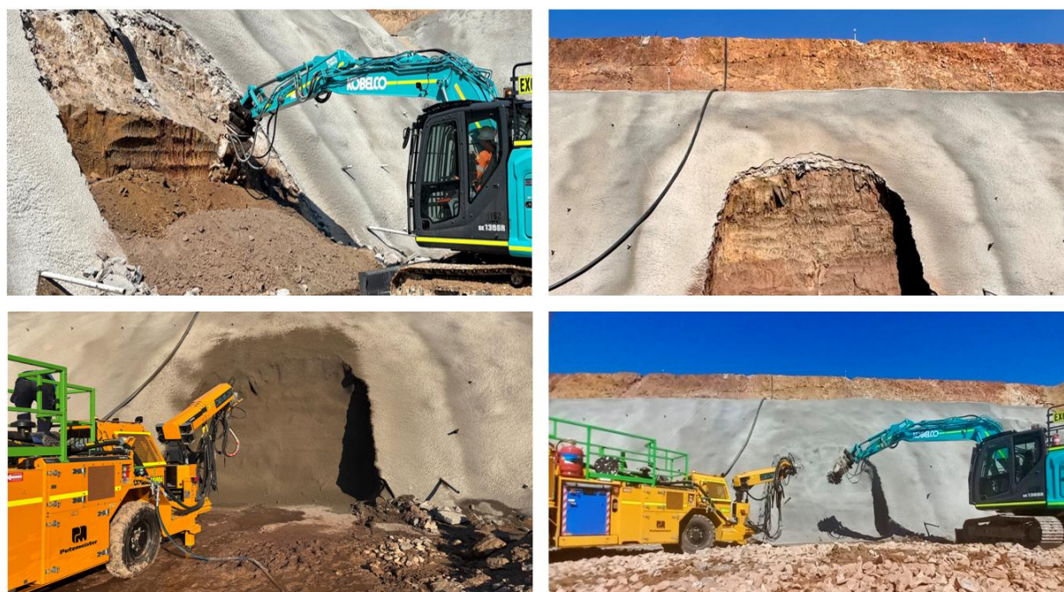
Figure 2: BP33 portal cut works (clockwise from top left): 1. Initial cut 2. Excavation of the portal completed 3. Fibrecrete applied to the face and brow 4. Fibrecreting of portal cut completed
