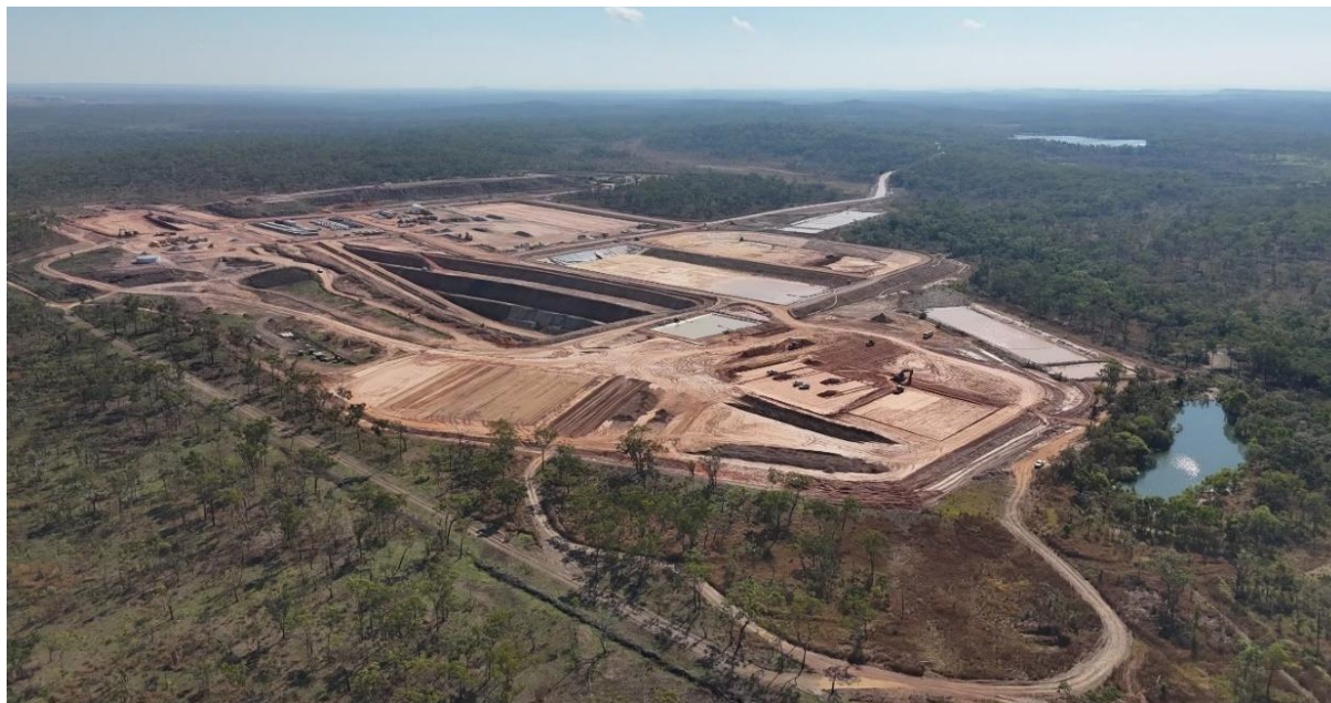
Figure 1: BP33 site overview with preparation of bulk earthworks pads for power station, primary fans and paste plant in foreground
