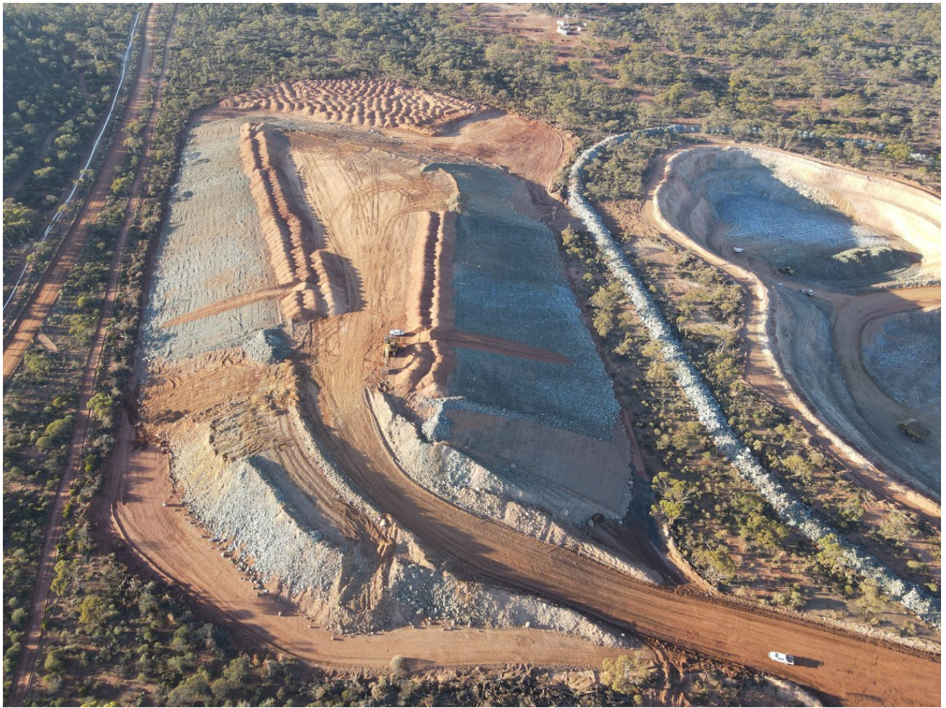
Figure 2: Rehabilitation of the waste dumps continues in parallel to the mining operations, as does construction of the final abandonment bund.
