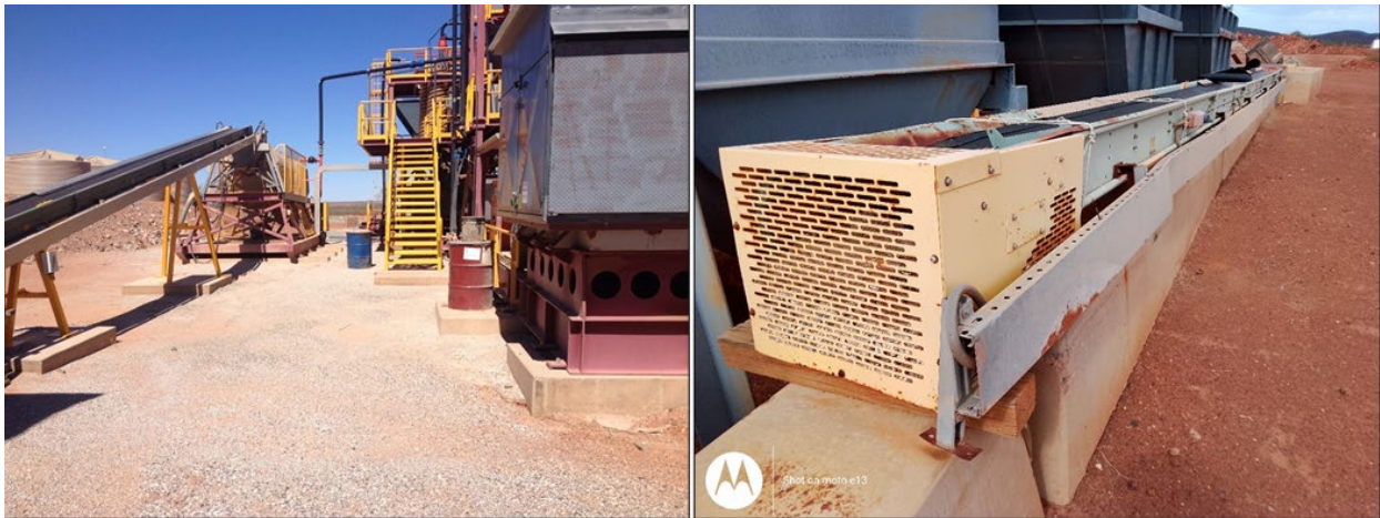
Figure 4: Rom Bin to Mill conveyor
