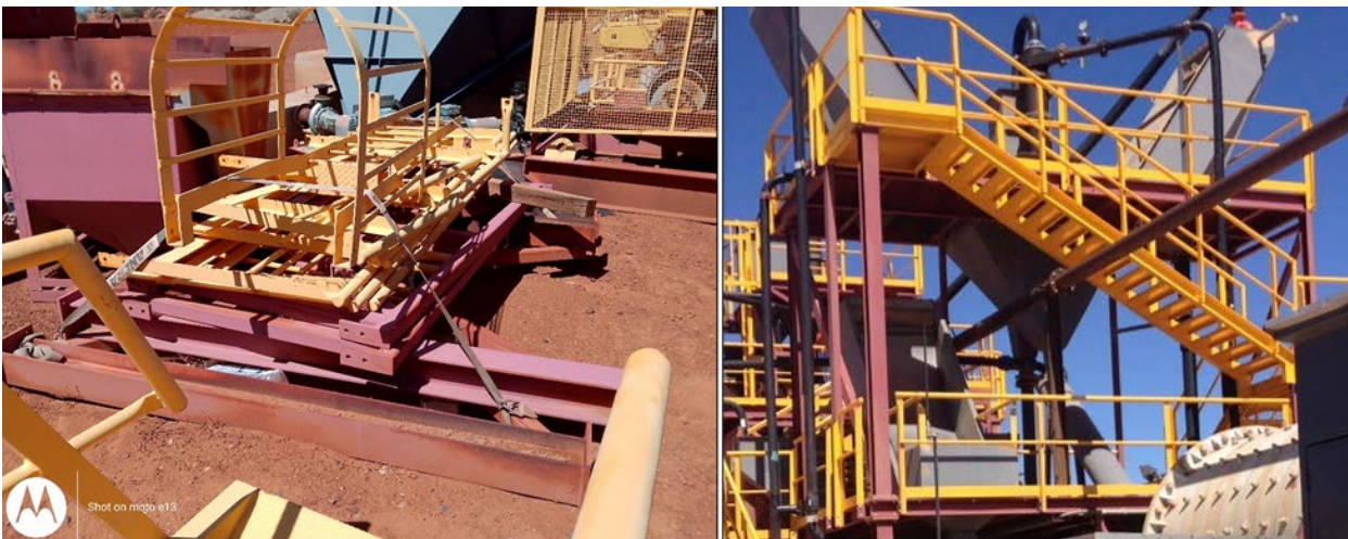
Figure 9: Screen and Cyclone Module
