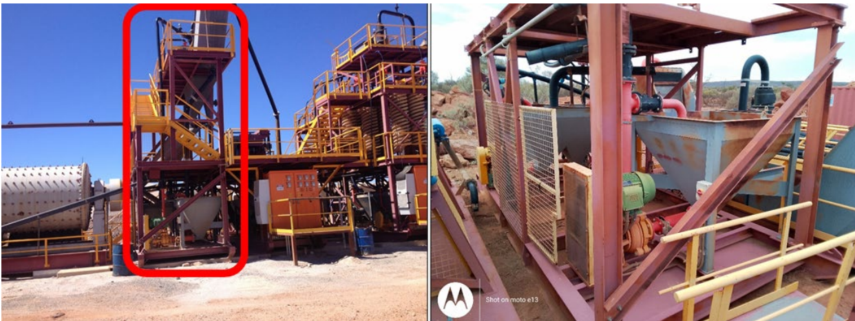
Figure 8: Screen and Cyclone Module
