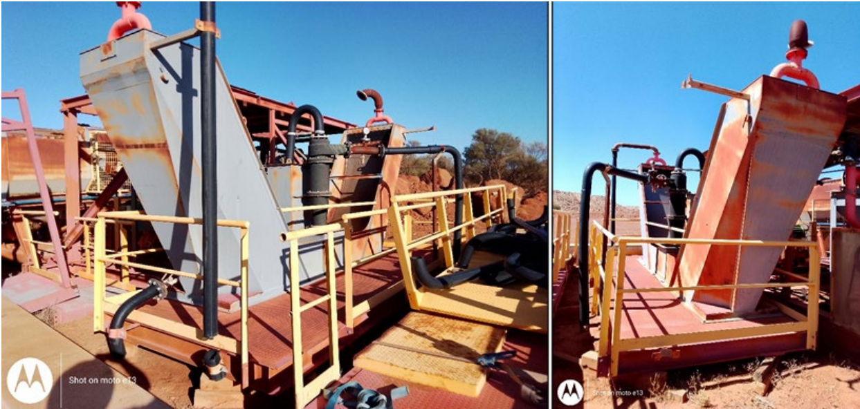
Figure 10: Screen and Cyclone Module
