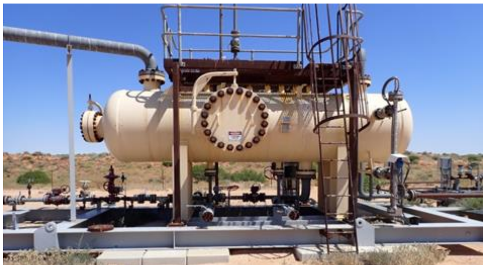
Figure 2: Gas/liquids separator in place at Vanessa facility
