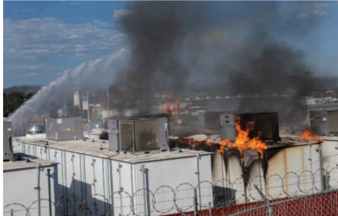
Escondido, California (September 2024): A BESS fire at a substation resulted in significant damage. The incident involved overheating of battery cells. Source: https://eticaag.com/thermal-runaway-in-battery-energy-storage-systems-bess/
