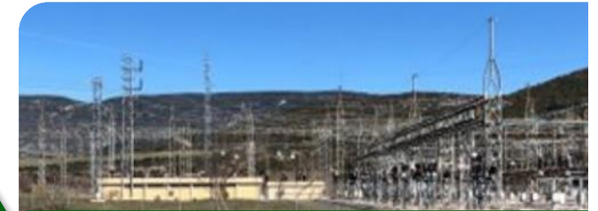
National Electricity Grid Substation in Sangüesa
