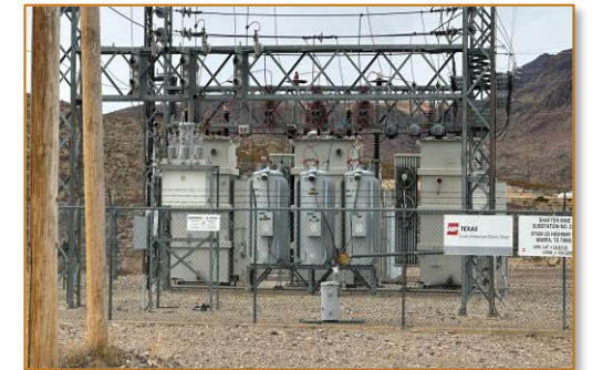
Shafter Electrical Infrastructure
