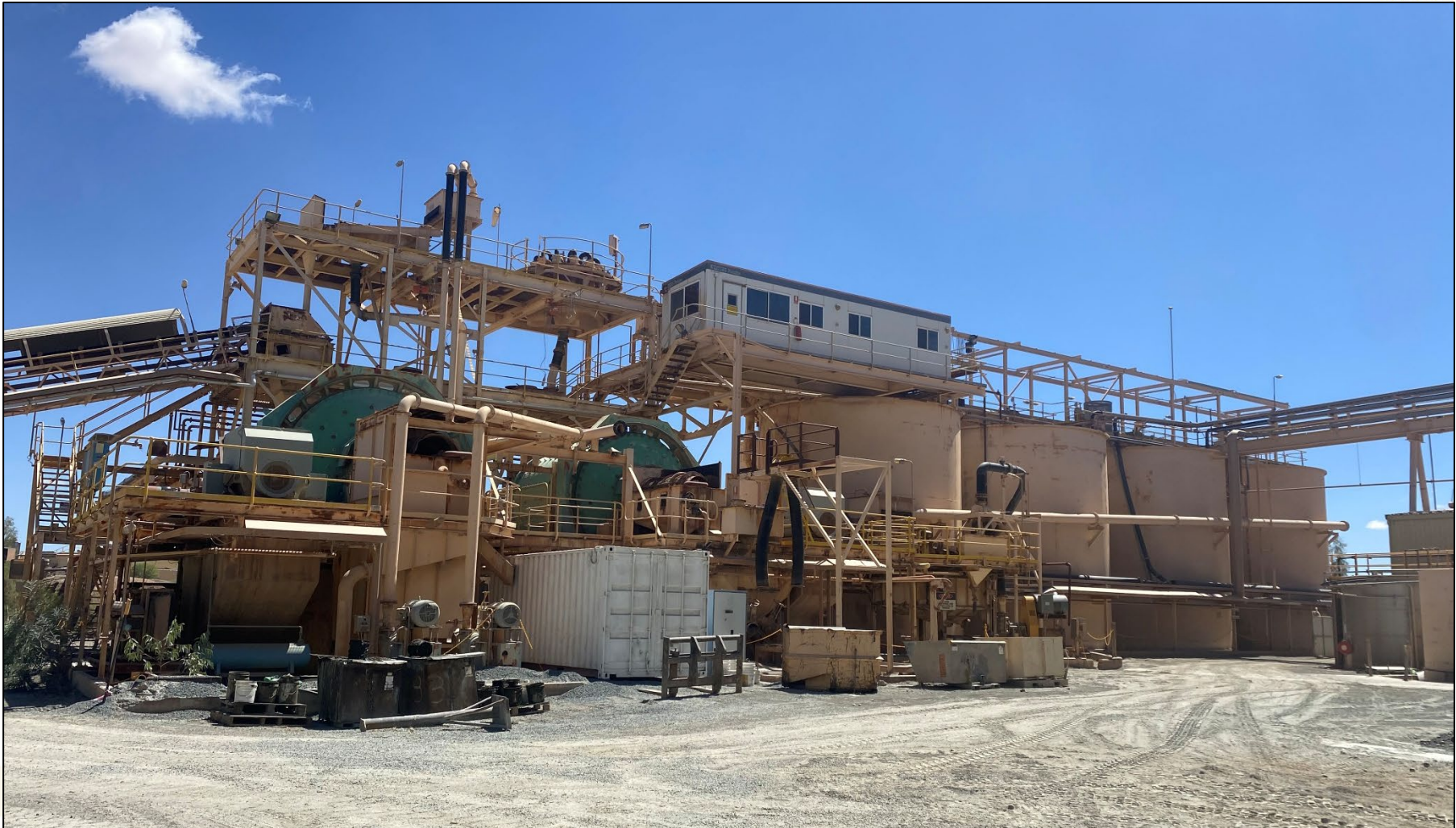
Figure 5: Plutonic processing plant 2 (PP2) showing SAG and ball mills, leach tanks and adsorption tanks
