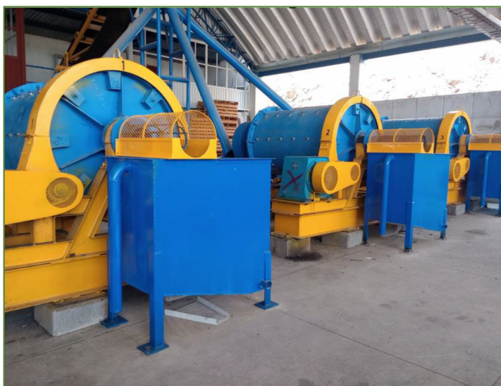
Figure 1 – Fully refurbished and dry commissioned Ball Mills 1 - 3
