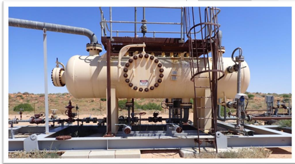
Gas/liquids separator in place at Vanessa facility
