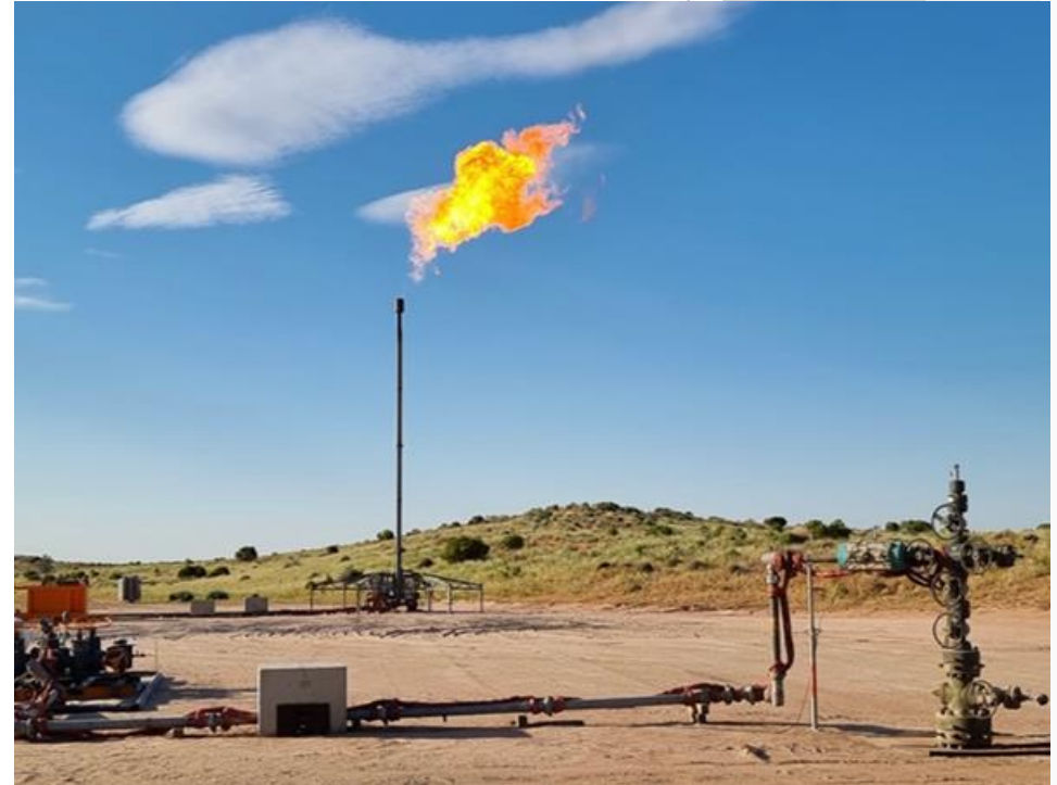
Gas flare at Kiwi-1 wellsite
