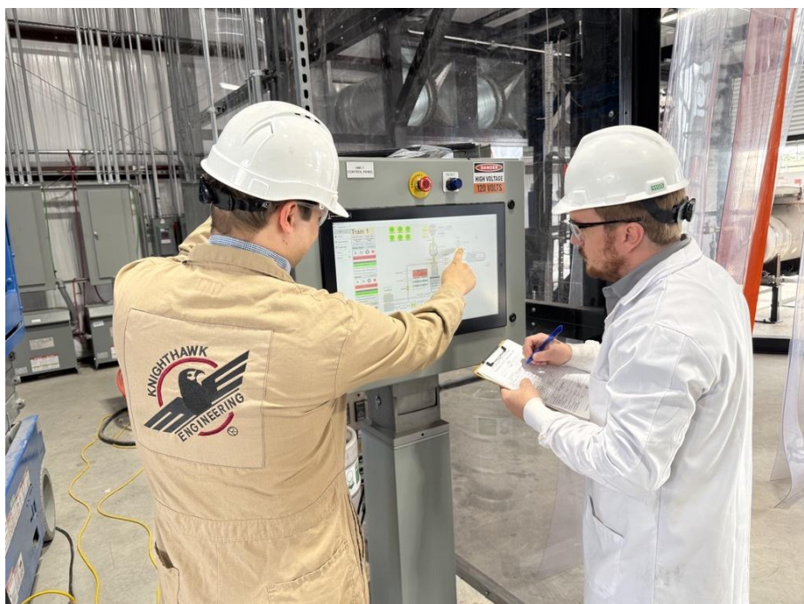
Figure 3: Integrated control unit to support technology automation
