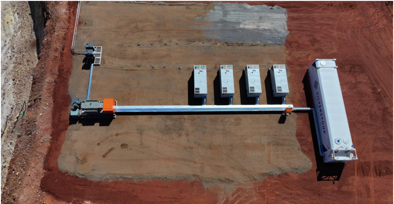
Figure 5 – Main and Pollard temporary power station
