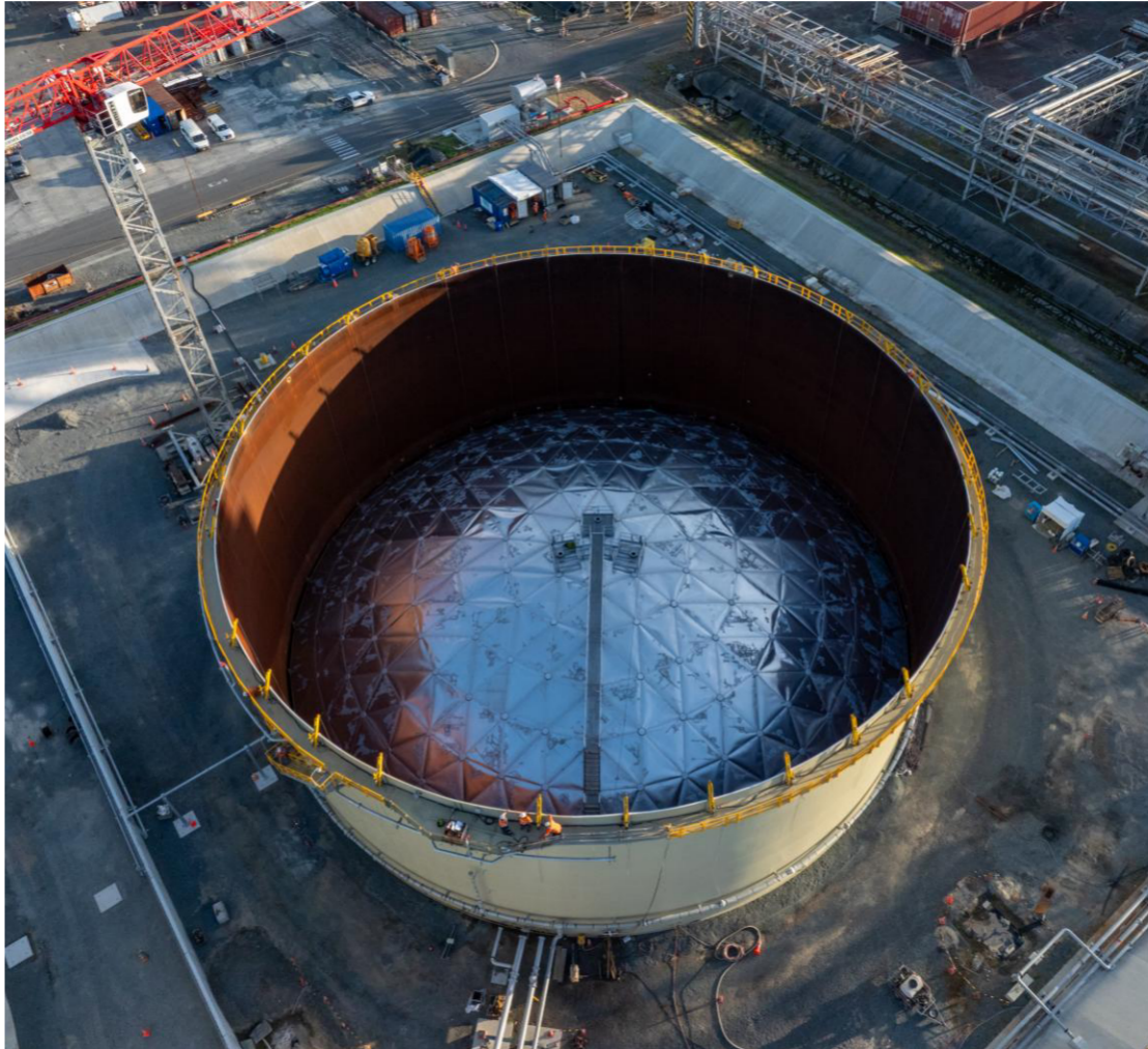
Jet Fuel Storage for Z Energy
