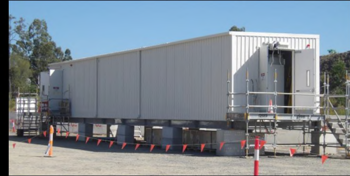
Pre-Assembled Electrical Switchroom
