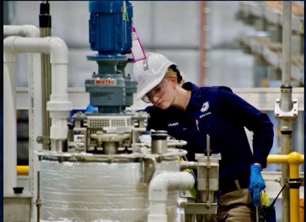
DEVELOPING THE WORLD’S LARGEST, SINGLE-SITE HIGH PURITY ALUMINA MATERIALS FACILITY IN GLADSTONE, QUEENSLAND
