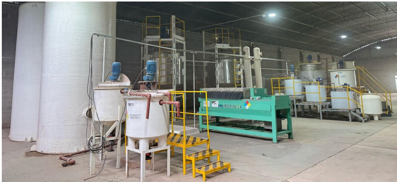
Figure 6: Pursuit's 250tpa Pilot Plant producing Lithium Carbonate in Salta, Argentina
