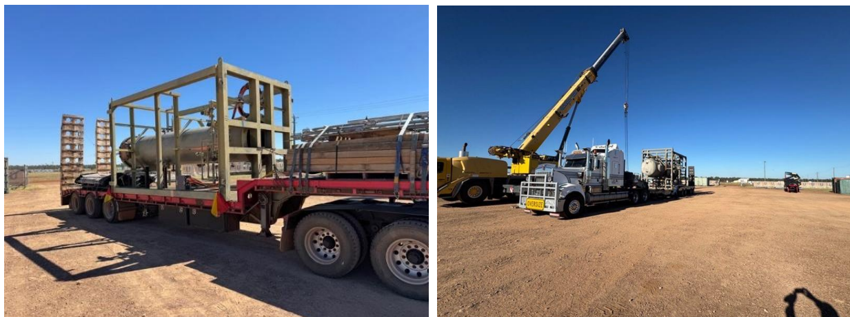
Refurbished units in Roma being loaded for transport to Carpentaria
