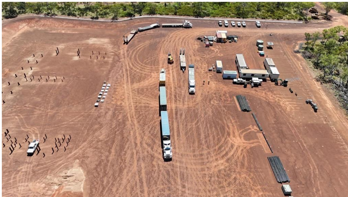
Aerial view of gas plant equipment being delivered to the Carpentaria site after trucking from Roma, QLD
