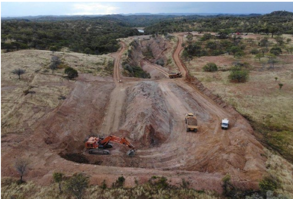
Figure 2: Excavation at Big Reef open pit showing exposed ore zone and historic open pit in background
