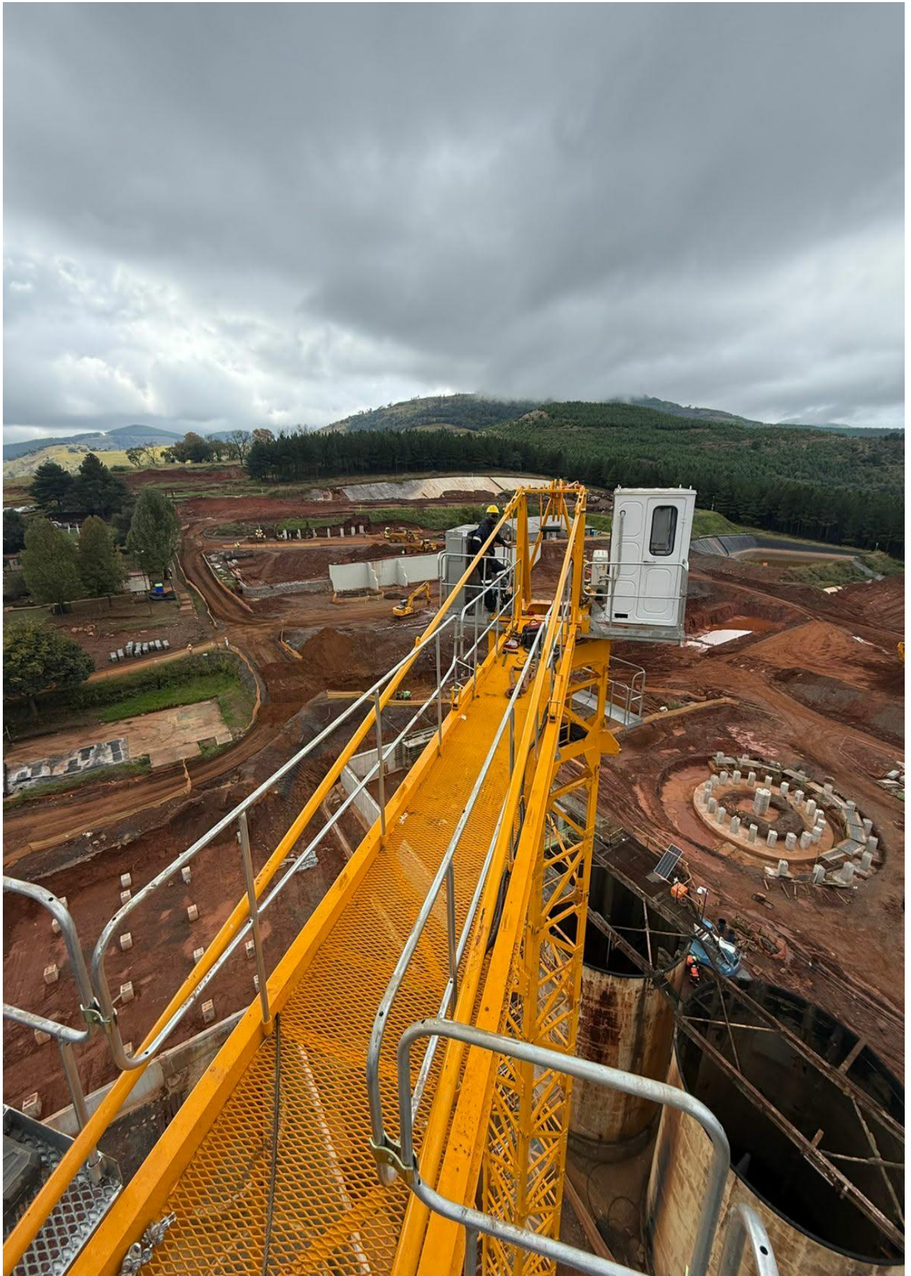
Figure 10 Stationary Crane now fixed in place at site for construction and maintenance
