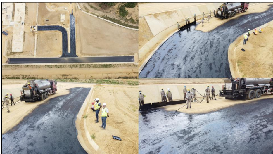
Figure 2 – Bitumen roads being completed at the Cabinda Phosphate Fertilizer Plant, in Subantando, Angola.
