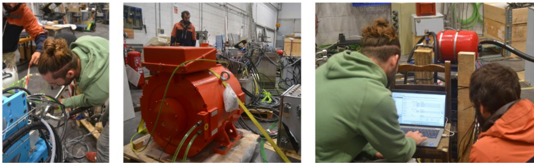
Integration testing of the electrical, control and cooling system prior to installation in the Electrical Module
