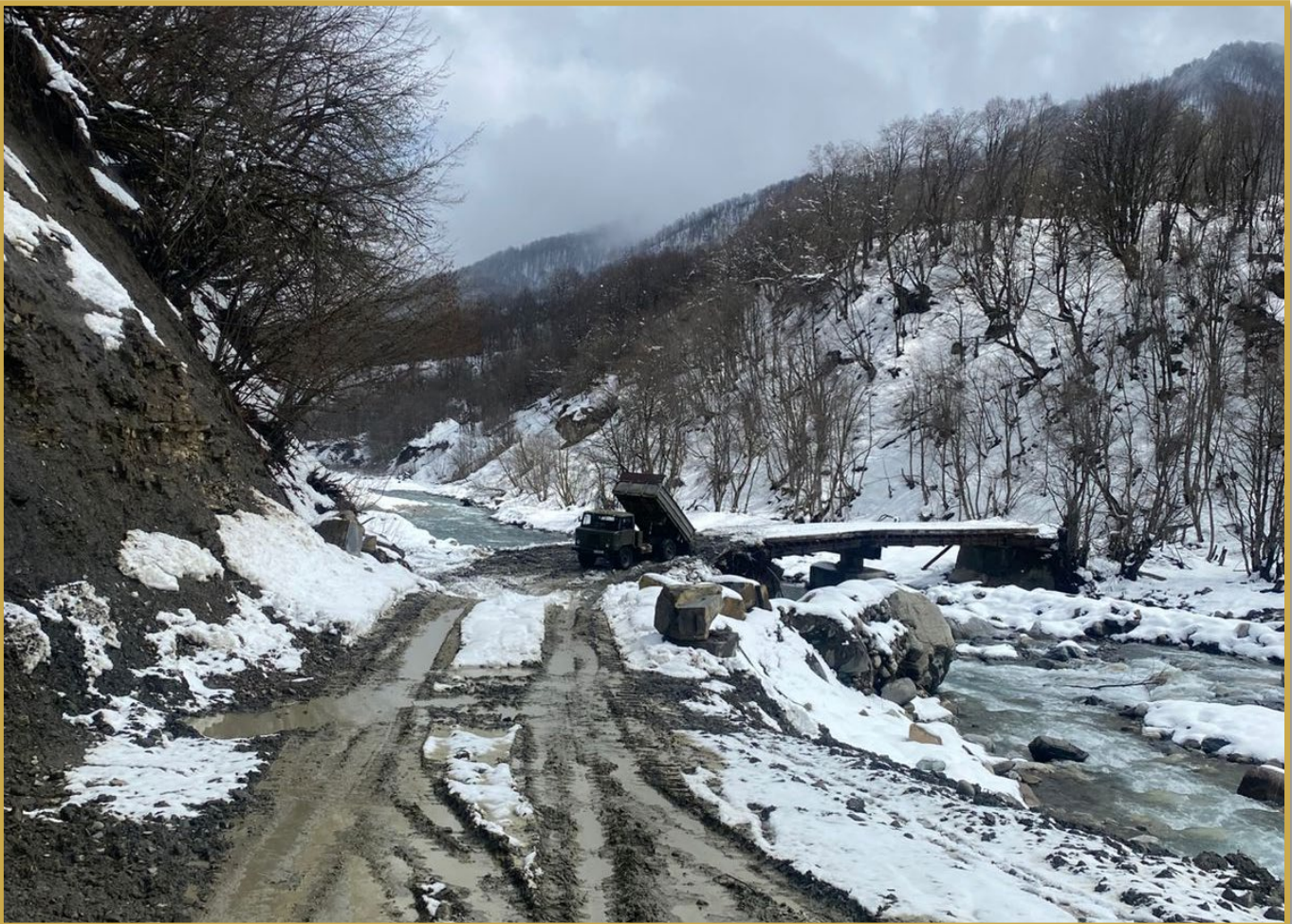
Figure 3 : Photograph of the road and bridge repairs for the access track to site (21 April 2026)
