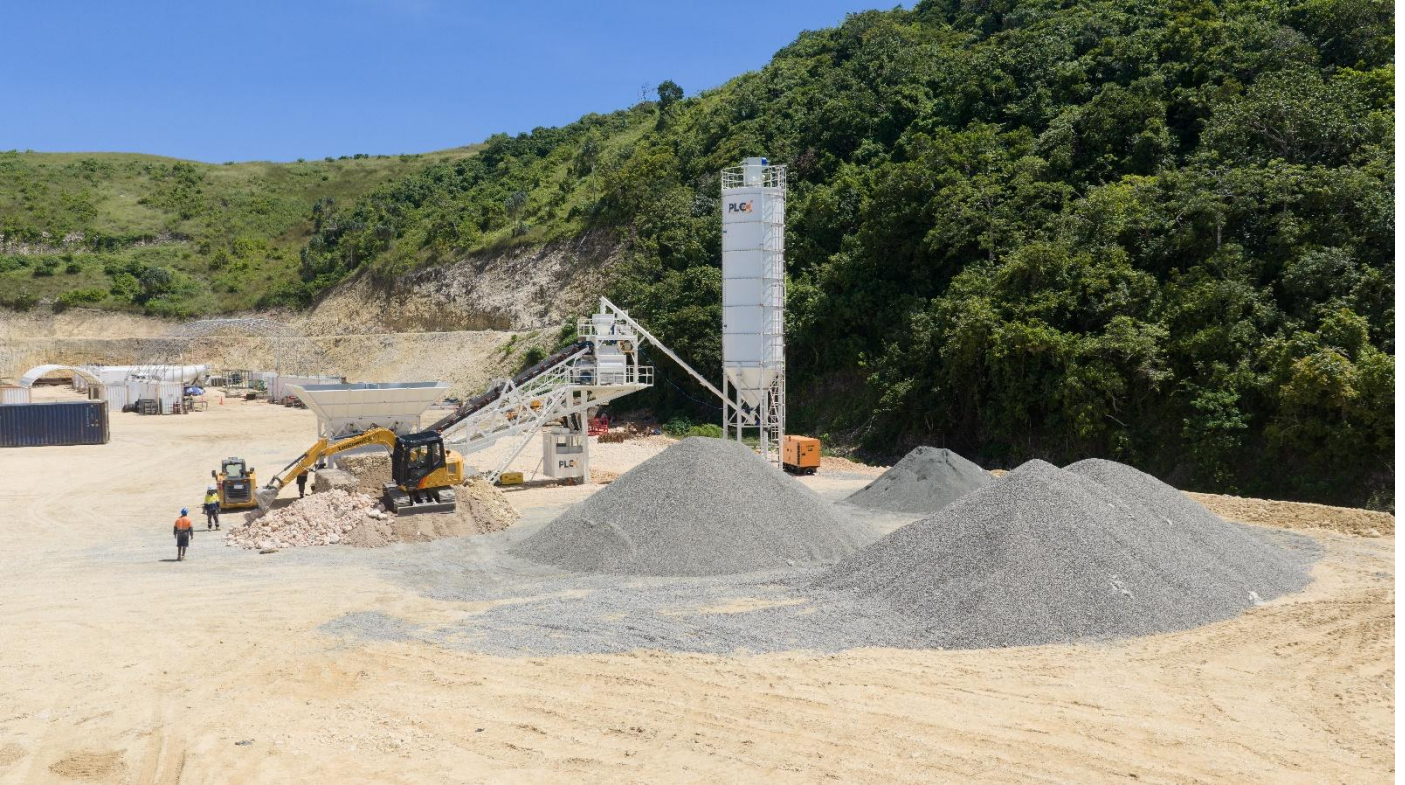
Image 7: Silos and other equipment in operation.
