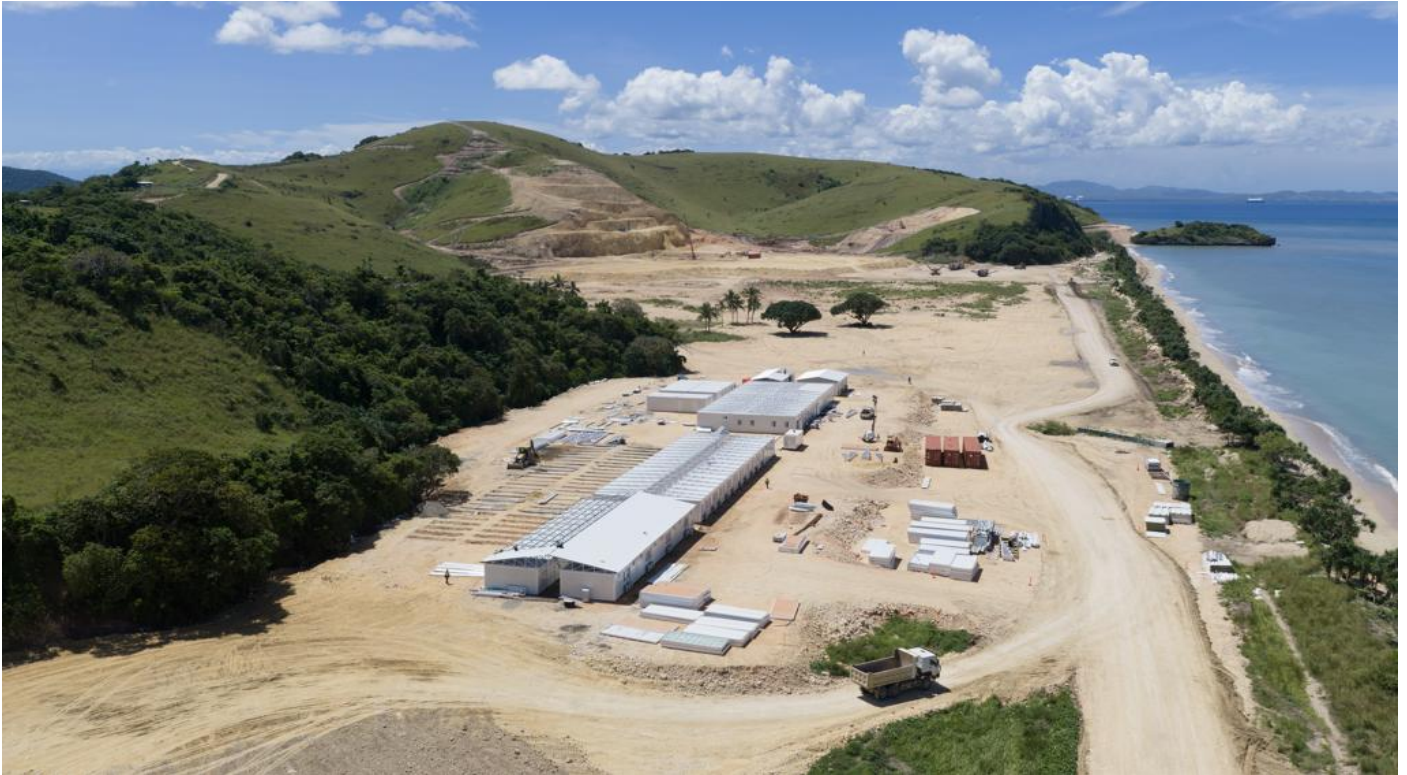
Camp infrastructure is now positioned to support the transition into structural phase operations.
