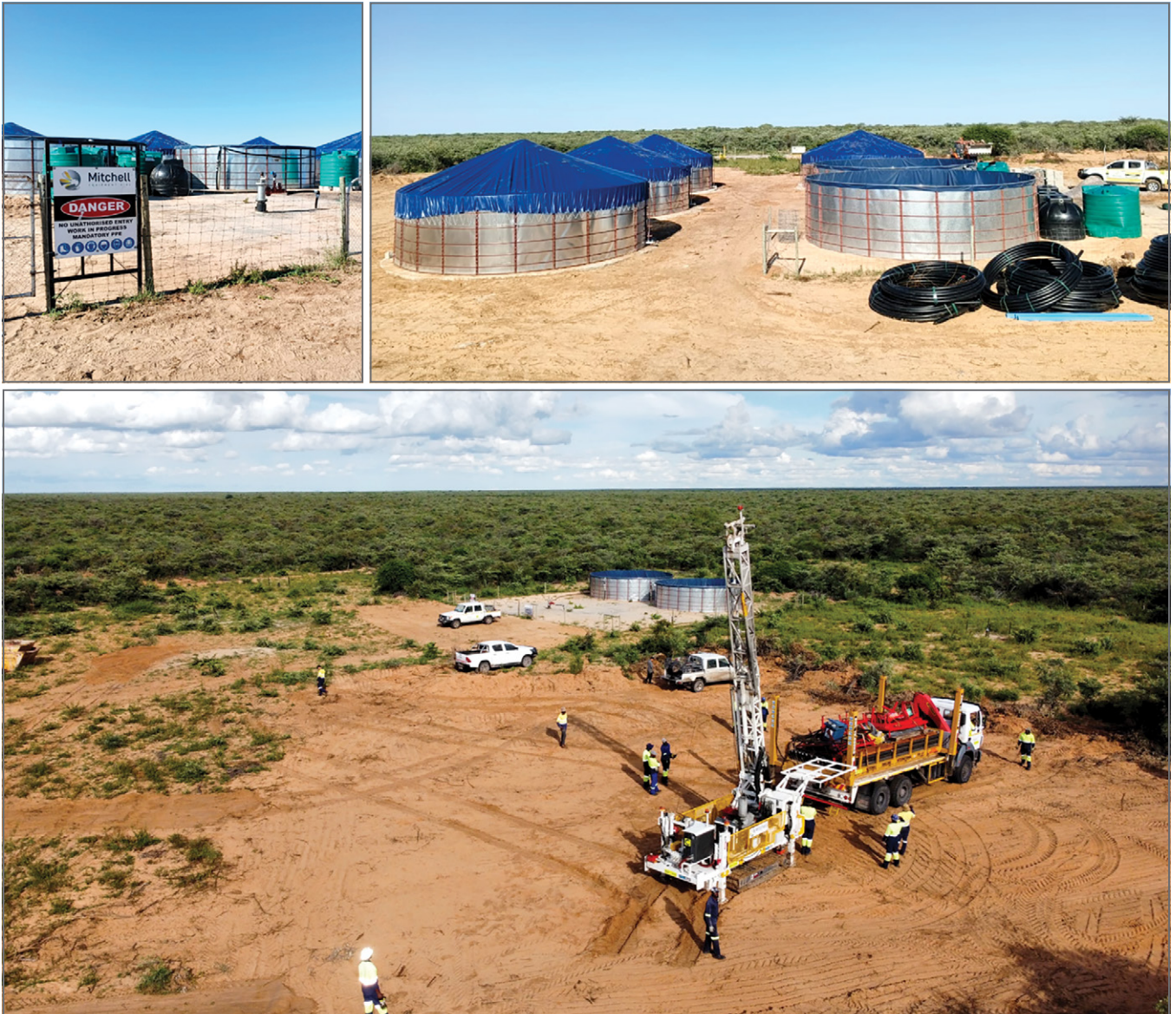
Figure 9: Ongoing well field drilling and tank farm construction for the demonstration plant at NCP
