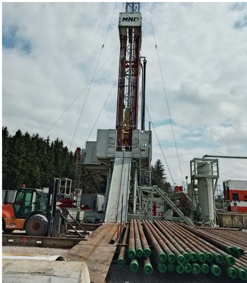
The MND Drilling & Services a.s. (MD-150) rig at the HOCH-1 drilling location
