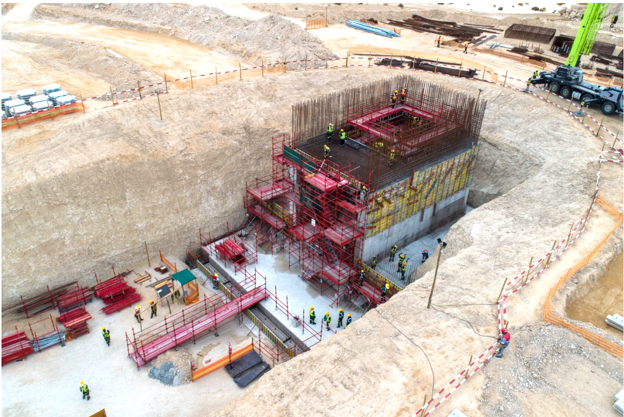
Figure 4: The primary crusher building foundations are complete with the first level walls complete.
