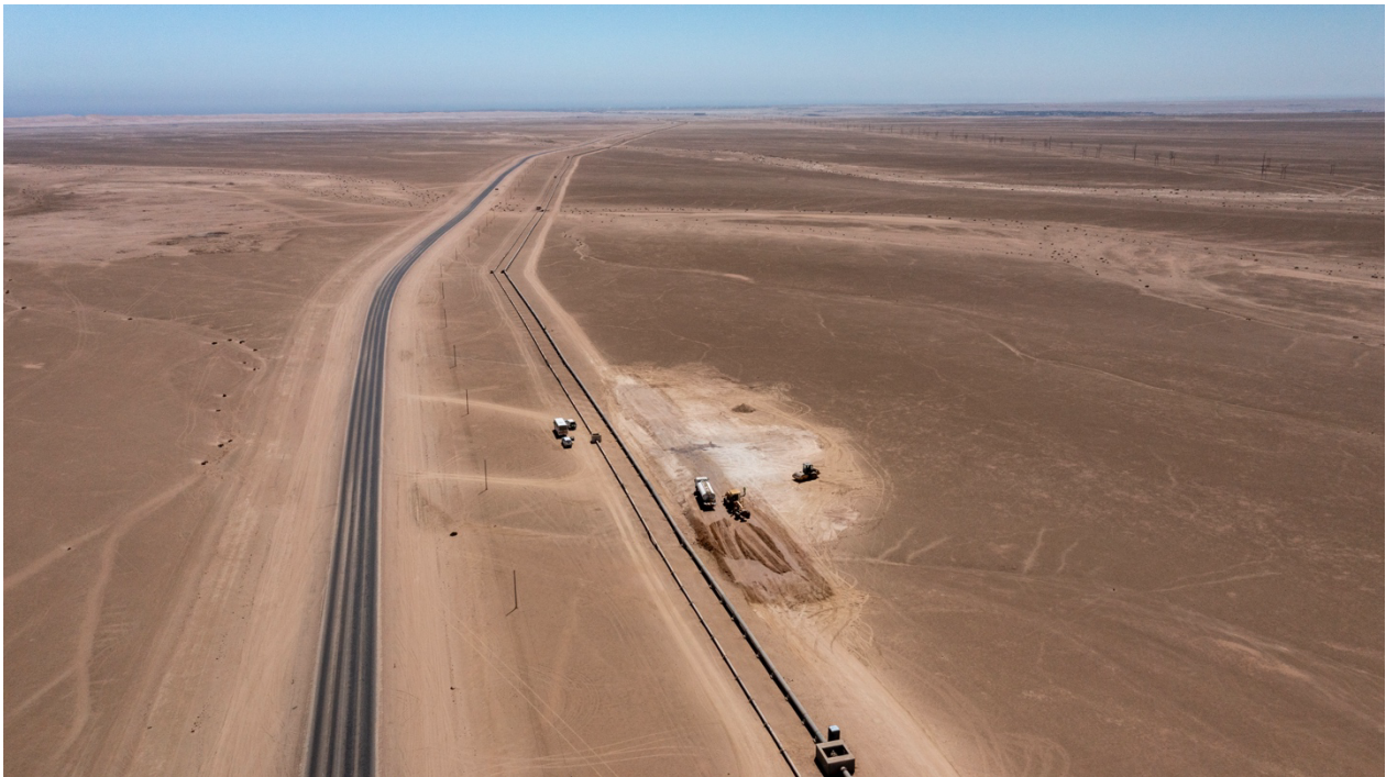
Figure 5: Excavations for the permanent water pipeline have commenced and are progressing in line with schedule.
