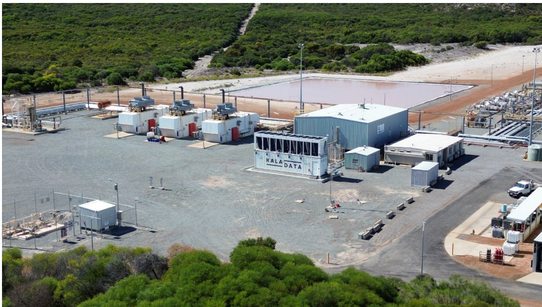
Photo 1: Photo of completed Dongara Data Centre 1MW Module at Cliff Head Plant site
