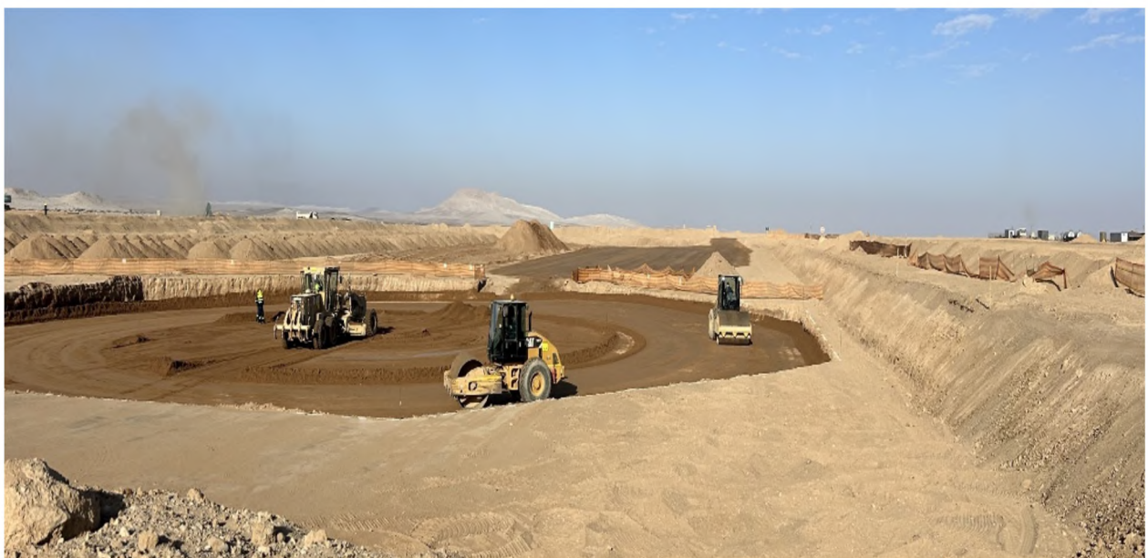
Figure 2: Bulk earthworks for the counter current decantation area at the Tumas Project.
