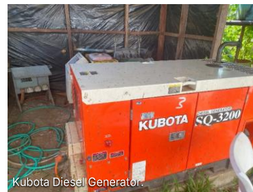
Kubota Diesel Generator.
