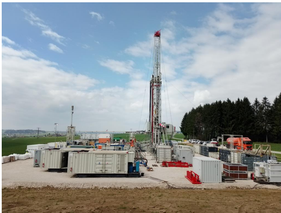
The MND Drilling & Services a.s. (MD-150) rig at the HOCH-1 drilling location prior to well spud
