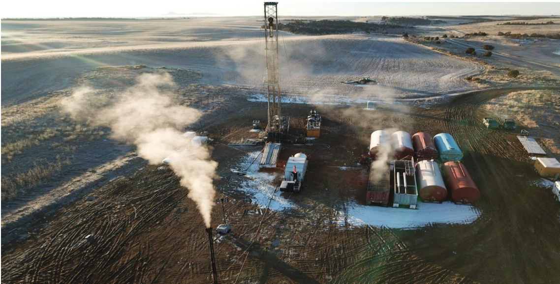
Jesse-1A flow test venting reservoir gases and helium through the flare stack in (Grand Gulf, 2022)
