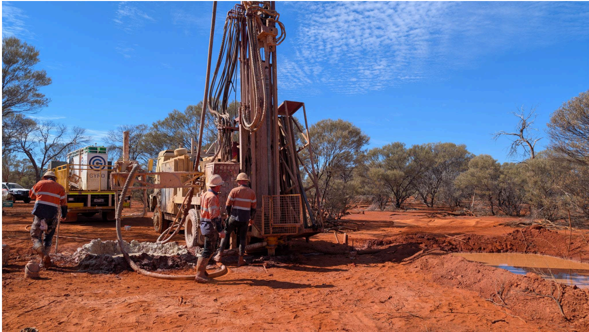
Figure 4 - Aircore drilling to refine location of Production Bores in Lake Raeside Paleochannel
