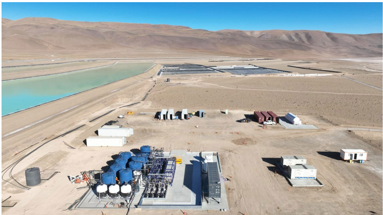
Figure 2. Completed nano-filtration plant.
