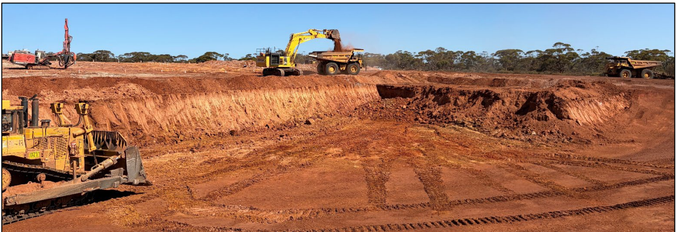
Figure 1: Mining activity in full swing during March 2026, looking southeast across the 315mRL and 310mRL benches.
