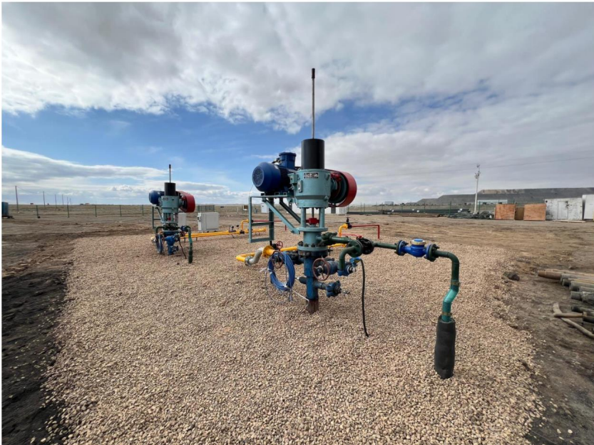
Figure 2 – Completed CBM Gas Production Wells at the Red Lake Gas field
