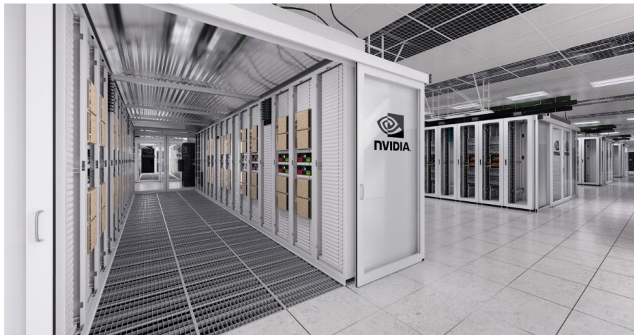
Pictured: An Nvidia data centre (NVDA.NAS, US$4.3 trillion market cap - source: Bloomberg).
