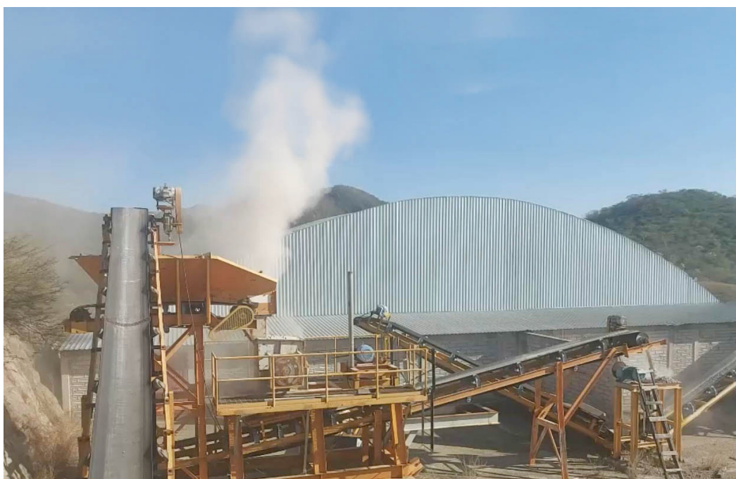
Figure 4: Tecomatlán Plant – Crushing Circuit
