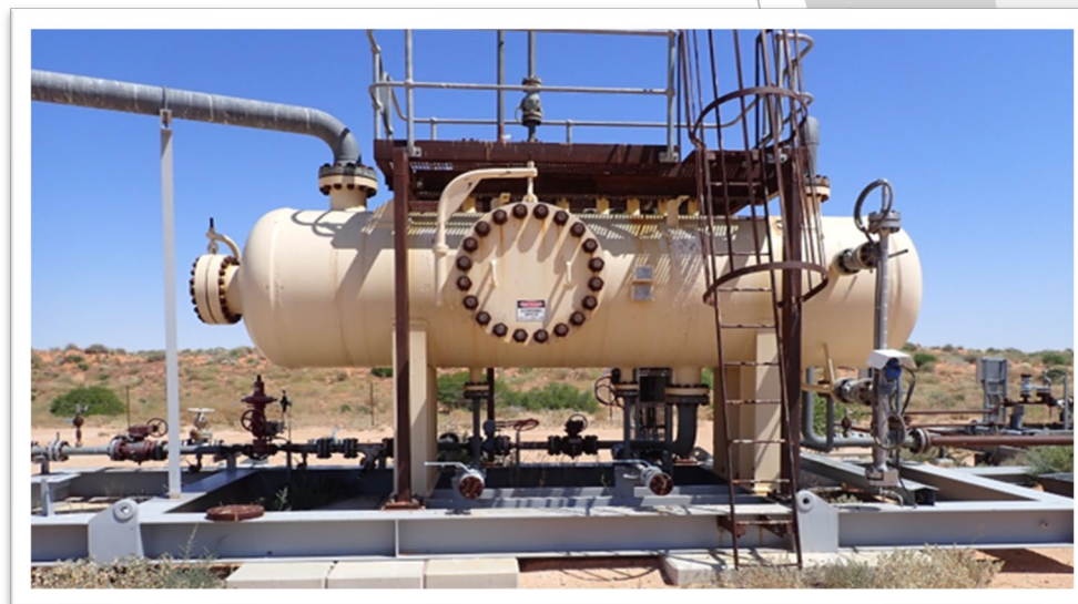
Gas/liquids separator in place at Vanessa facility
