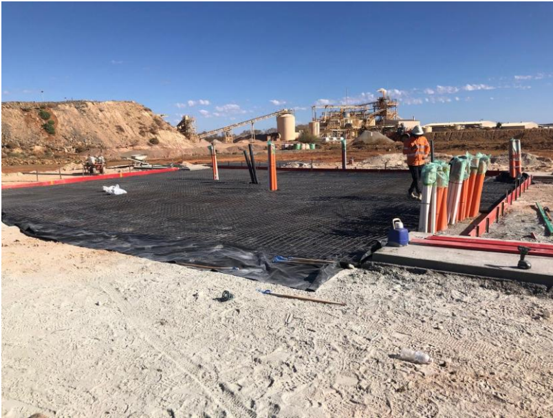
Figure 4: Ore sorter pad with electrical supply conduit.
