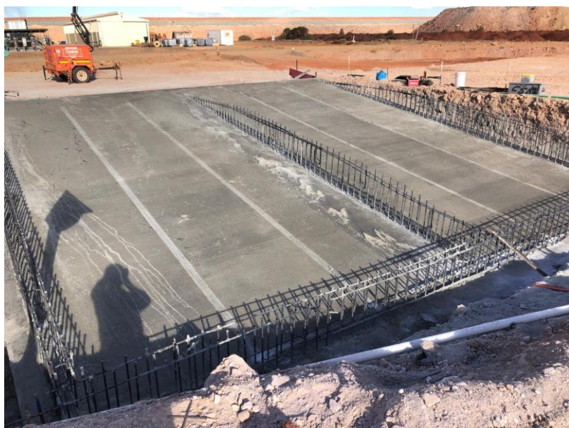
Figure 6: Wash plant sumps.
