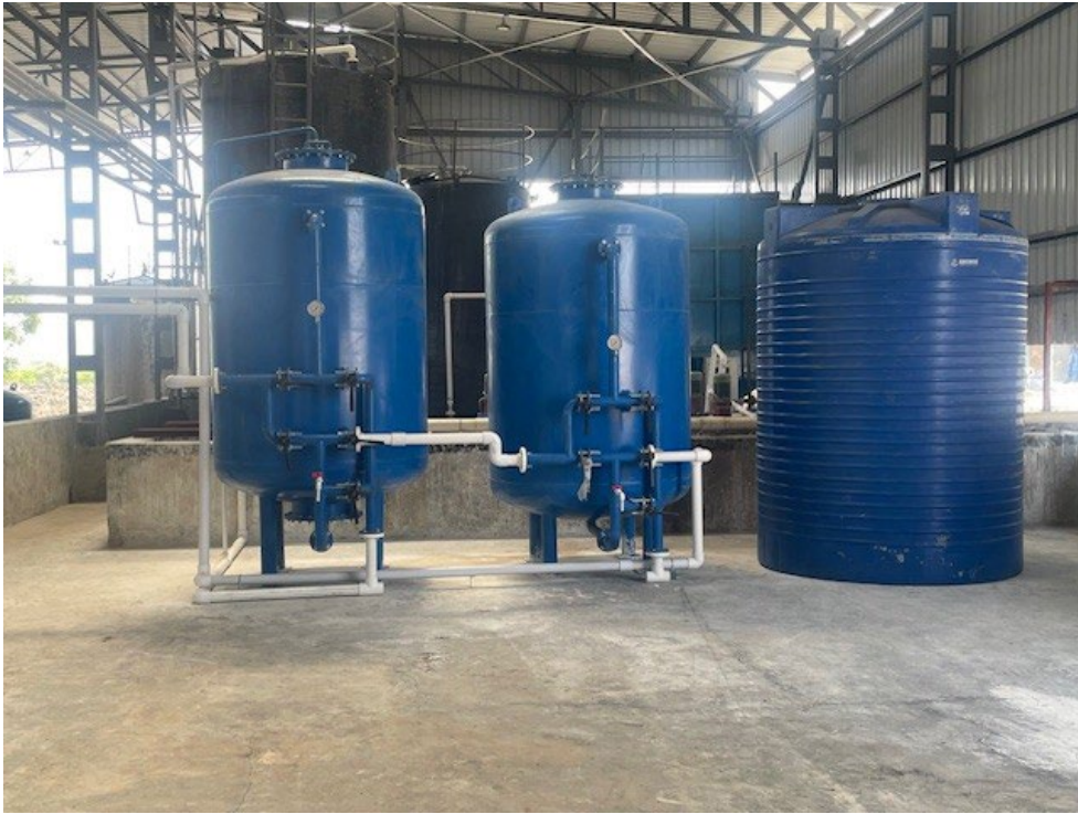
Figure 4 – Part of the effluent treatment plant that provides for 95% recycling of water
