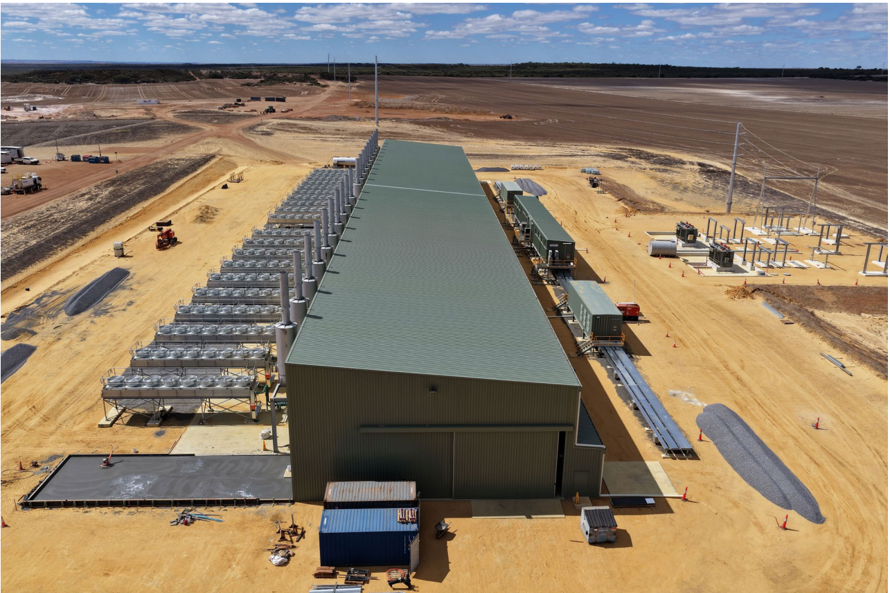
Power Station Package and 15 km Overhead Power Line
