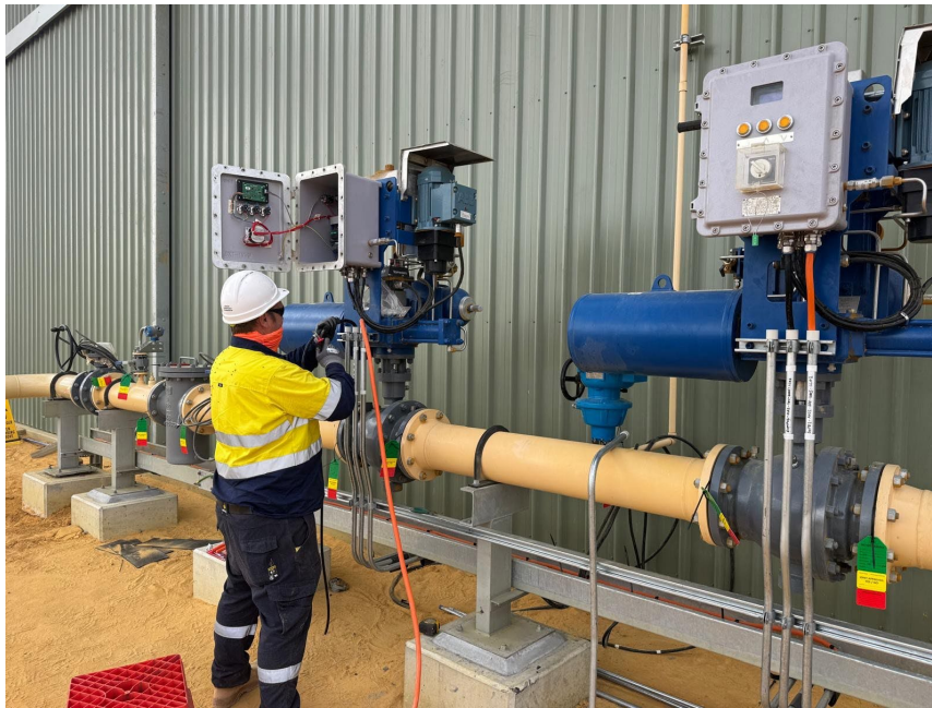
Termination wiring at the Power Station Inlet Gas Valves
