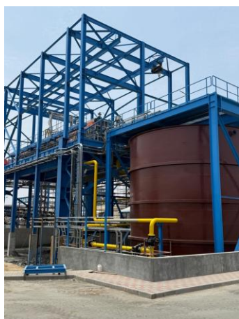
Image: New tailings filter press building & tailings tank
